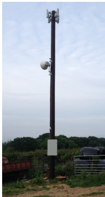
Figure 3: Example of a macro cell installation (this mast is 15 meters – masts can be as high as 30 meters).
