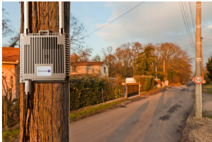
Figure 2: Example of a small cell installation.
