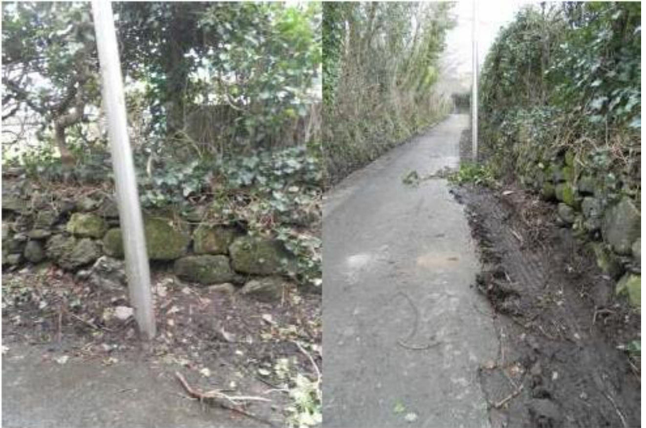
Figure 1 Struck lighting column number 2
